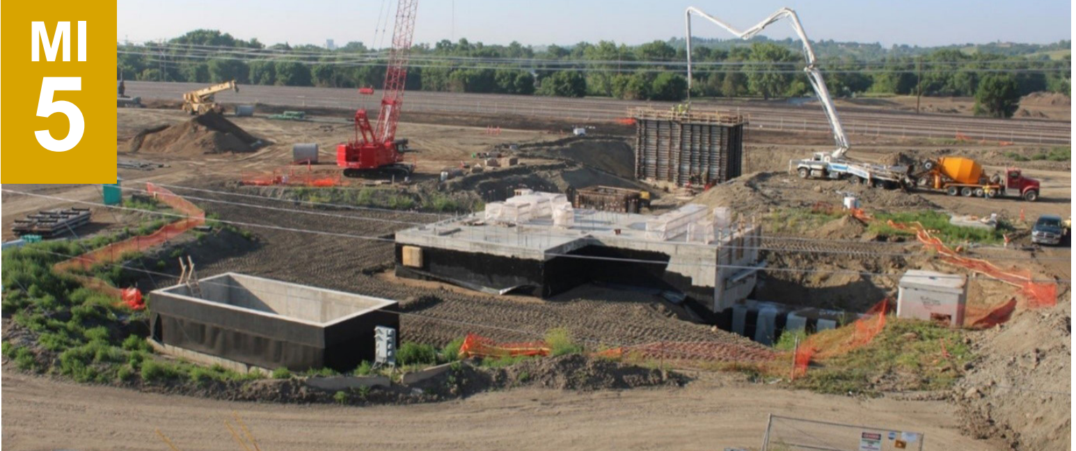
Booster Pump Station Foundation (foreground), Storm Water Pump Station (middle ground), and Pump Discharge Chamber (background)
