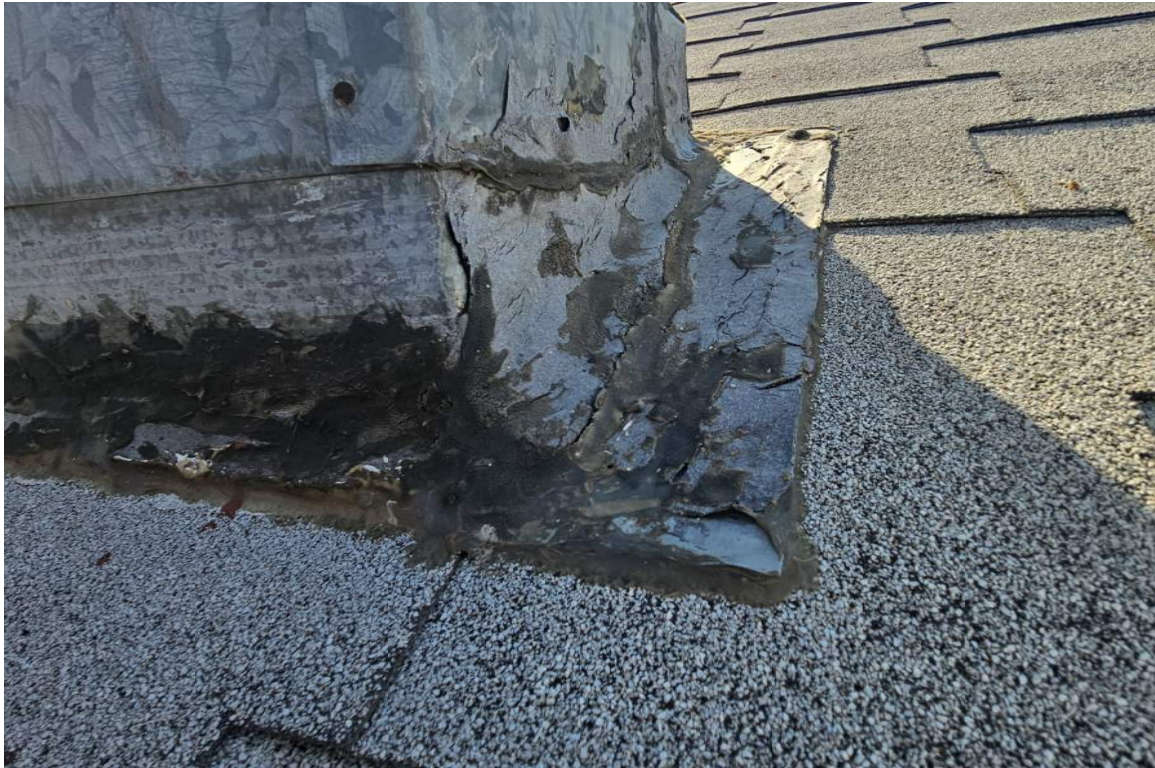
Photo 2 Single garage chimney sealant.
