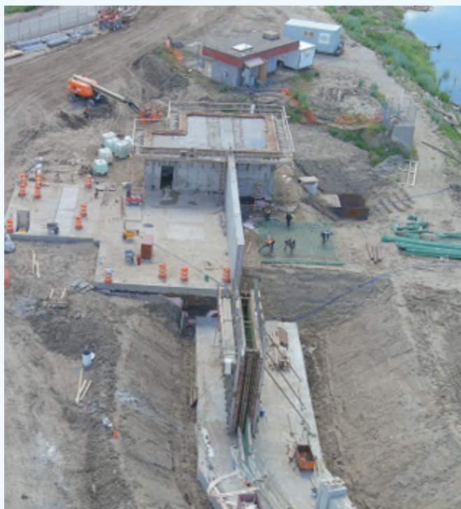
▲ 7th St Removable Closure & Floodwall
